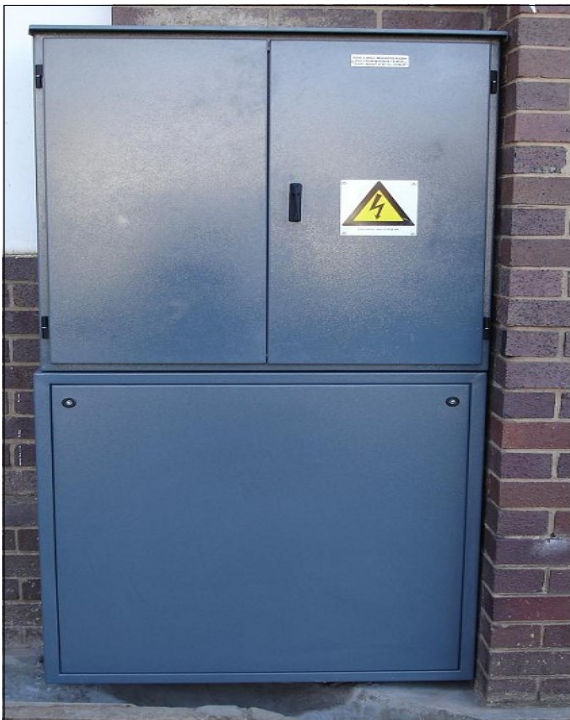
Outdoor Cable Box
