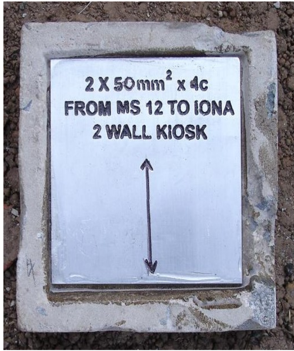
Straight Run Cable Route Marker
