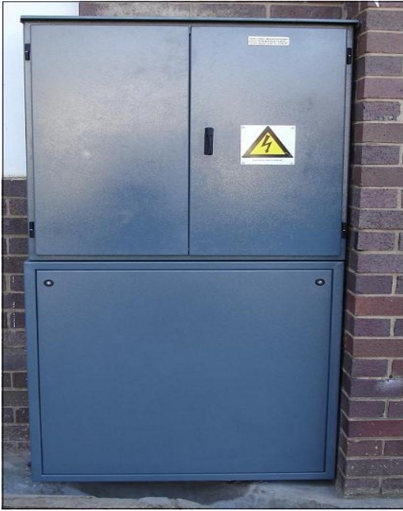
Outdoor Cable Box
